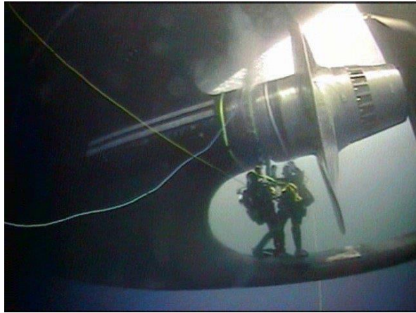
At McMurdo, divers repair a leaking shaft seal on the Polar Star.
