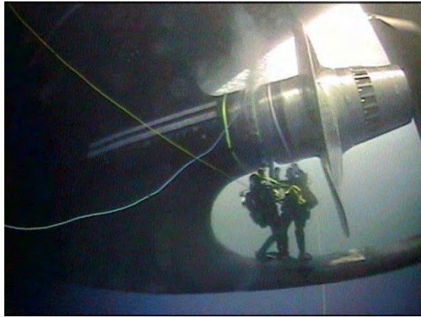
At McMurdo, divers repair a leaking shaft seal on the Polar Star .
