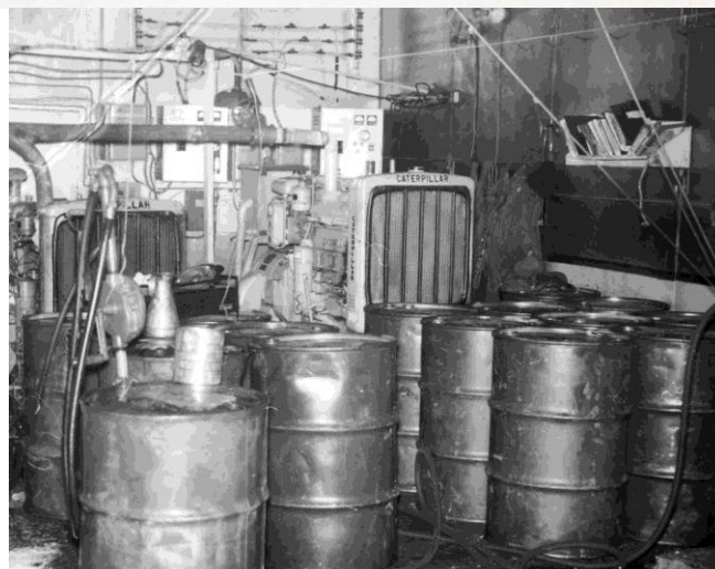
Our Diesel Generator
